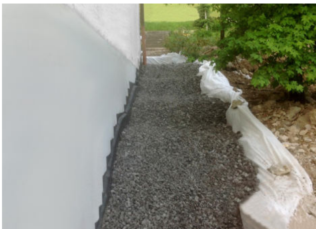
Filling in the working pit and compressing GEOMATERIALS Foam Glass in layers
